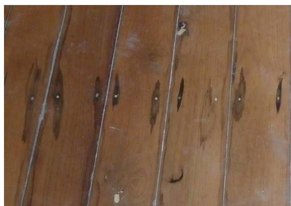
In this old hoop pine floor, the staining is extensive.
