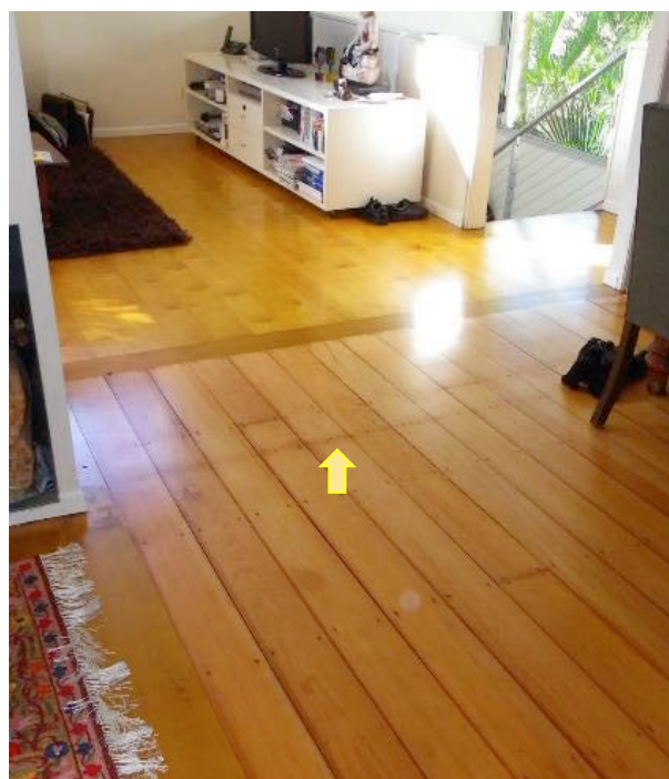
At the top of the photo the floor was not resanded and coated due to the architectural break. The resanded and coated flooring in the lower section of the photo had been tinted in an attempt to match. If it had not been tinted the boards would have looked 'white' in colour. Note also the arrow indicating a colour difference where a past internal wall had been present.
